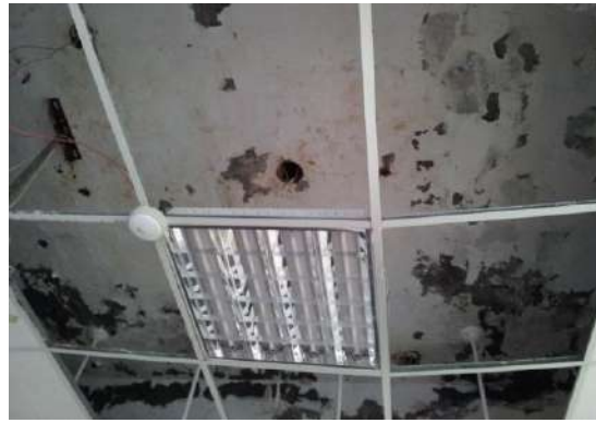
輕鋼架變形嚴重
